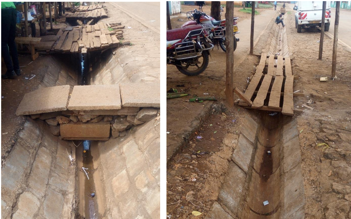
Figure 7: A section of lined drainages opposite the Ruiru Level IV hospital and the road connecting the Market to the Sub County offices
