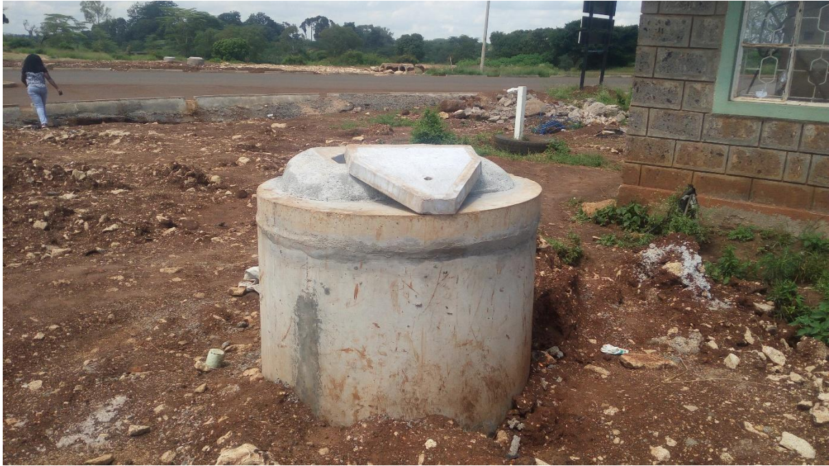
Figure 15: Man-holes along the trunk sewer line from the Tatu City Development
