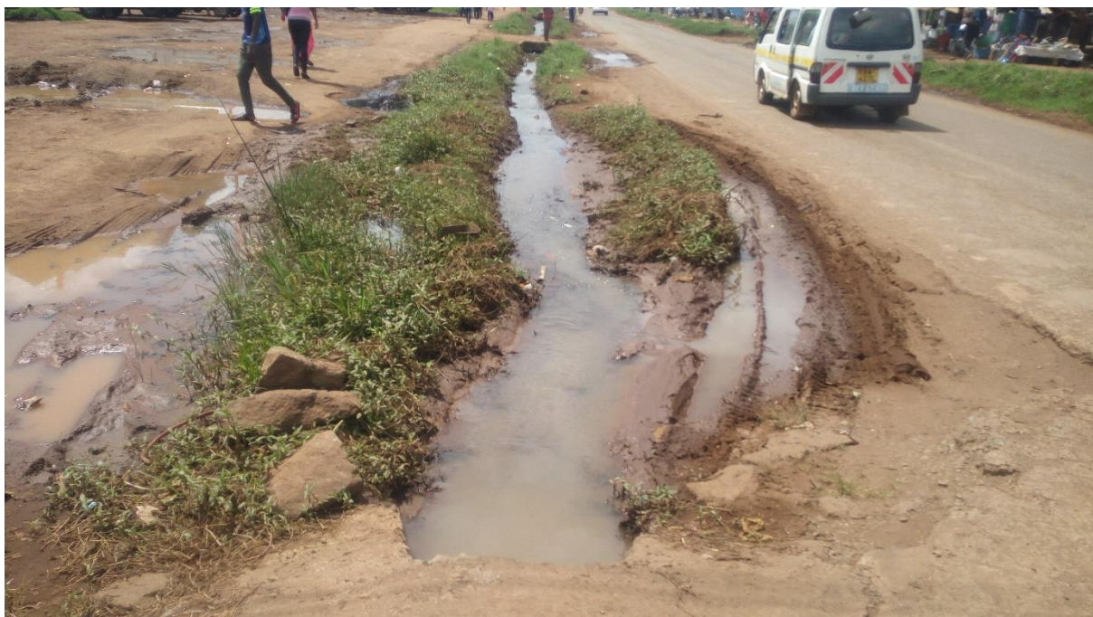
Figure 9: A clogged section of the storm water drain along Ruiru-Kamiti Road
