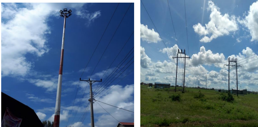
Figure 7: Electricity, Reticulation and Street Lighting in Limuru Municipality
