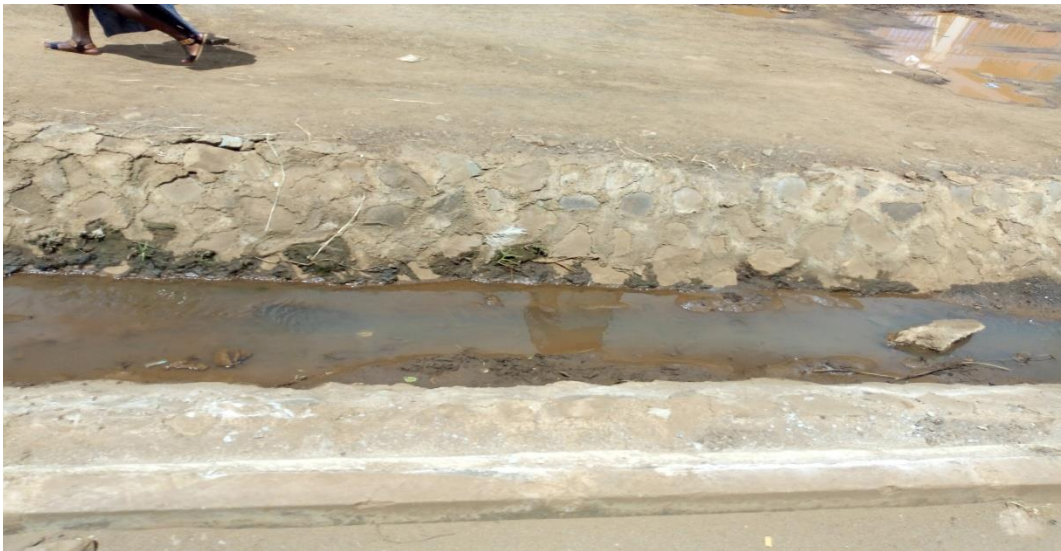
Figure 3: Storm Water Drainage in Kiambu Municipality
