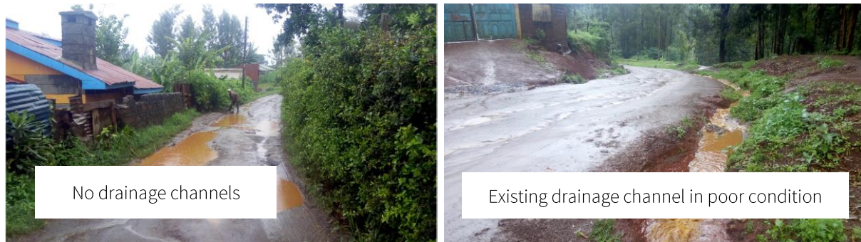
Figure 8-2: Storm water drainage channels in Gatundu
